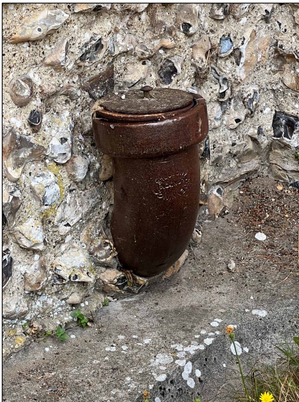
The stoneware pipe on the south side of St Mary's church Breamore.
