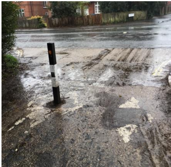
Southampton Common: The junction at Cemetery Road, Hill Lane & Raymond Road, enlarged and reinforced with concrete. Photo: S Hanna
