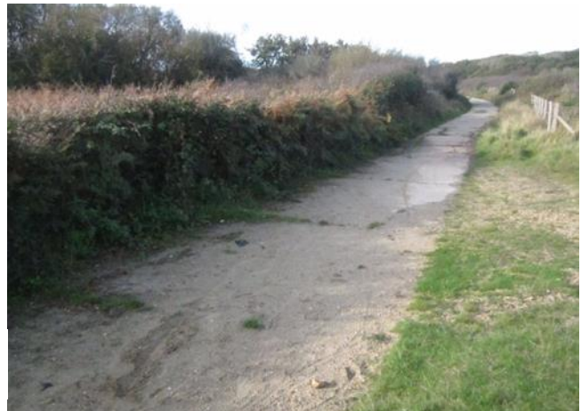
Roadway for access to embarkation beach at Lepe, note concrete laid in segments. Photo: S Hanna
