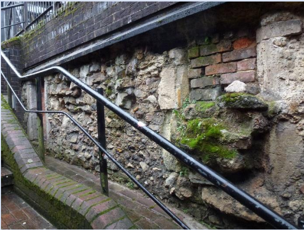
Fig. 1 A flight of stairs built in 1989 give access to the vault via the eastern doorway. Two blocked windows are shown.
