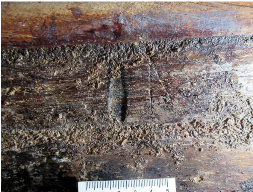
Fig 17 Burn mark on bedchamber tie beam, Truss E.
