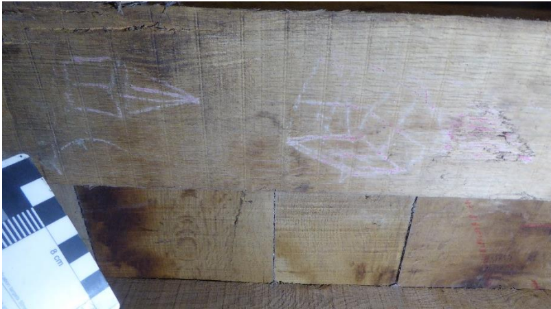
Fig 8 Passageway ceiling, modern chalk graffiti
