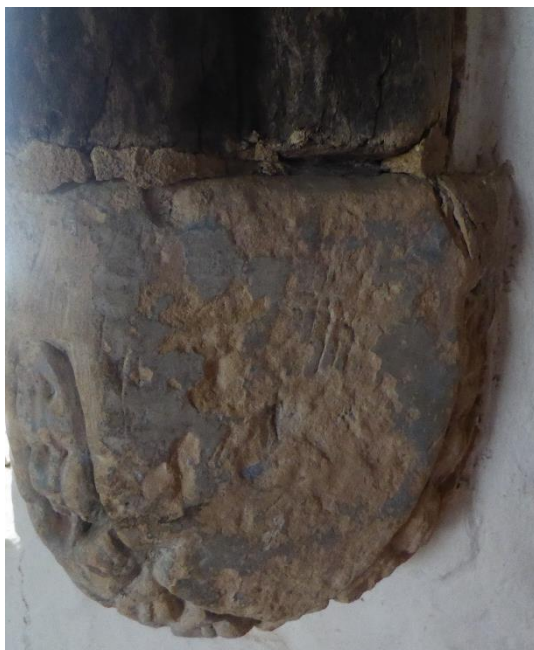
Fig 7 Inner room, north corbel, scratches and paint
