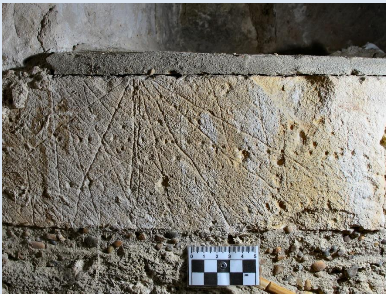
Scratched lines on stone sill of aumbry, to north of east window on second floor
