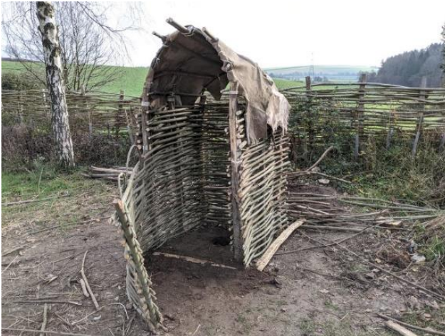
Operation 'Fix the Loo' 2022 - The Iron Age 'loo with a view' before and after.
